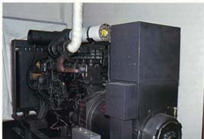
The standby diesel generating set.
